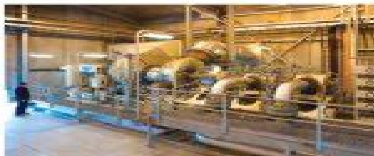
C16 Gas Compressor
